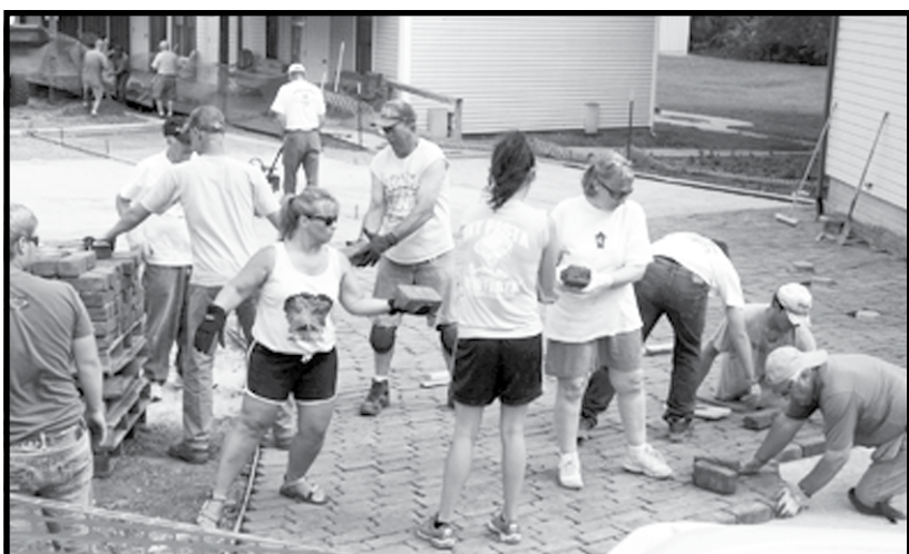
Volunteers from Our Savior Lutheran Church in Wayne work in brigade format to lay each brick by hand.
